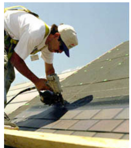
Figure 4.27 Roof-mounted Residential Solar Collectors, Image by Department of Energy
