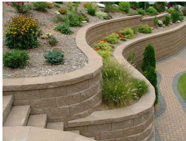
Figure 801-A: Retaining walls shall be benched, or terraced, so that no individual wall exceeds a height of six feet.
